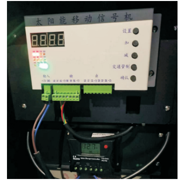
Sub controller (Channel 1)
