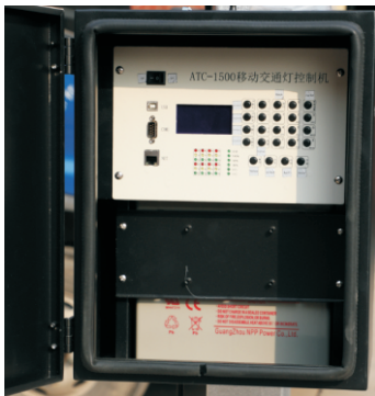
Main Controller (Channel 1)
