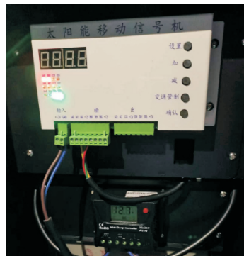
Sub controller (Channel 1)
