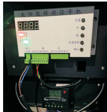
Sub controller (Channel 1)
